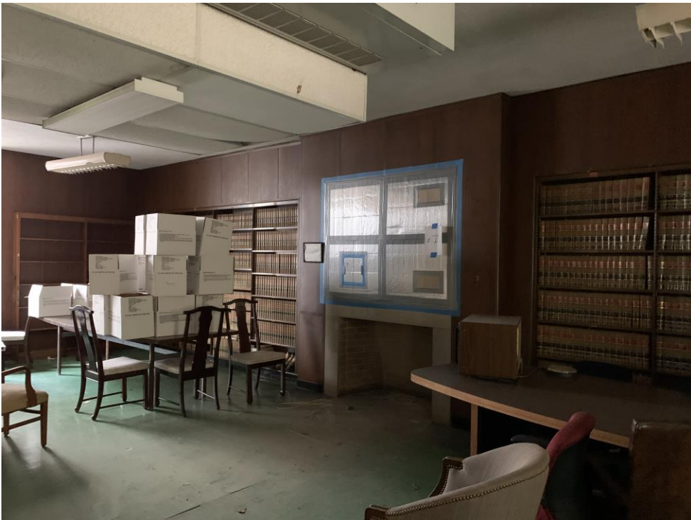
Interior view of Library looking northwest with fireplace on north end wall 21 of 23
