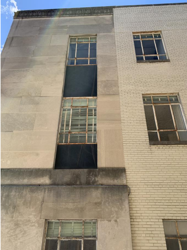
View looking west (skyward) showing east elevation at end of first bay where stone meets brick walls 7 of 23
